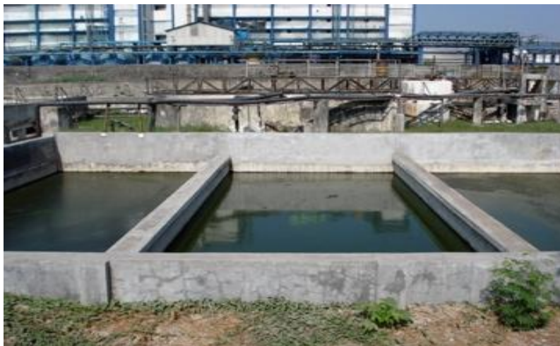
Figure 1: Treatment tanks for BRC's IMAET biotechnology treatment
